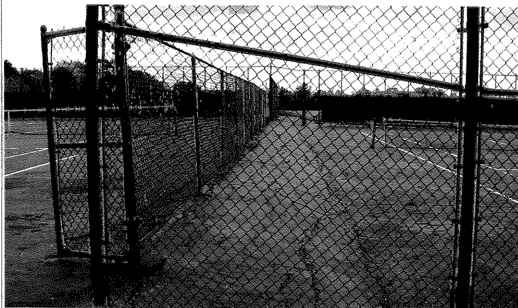
Improper footwear, water accumulation and fence climbing are just a few of the preventable causes of damage to courts and fences.
